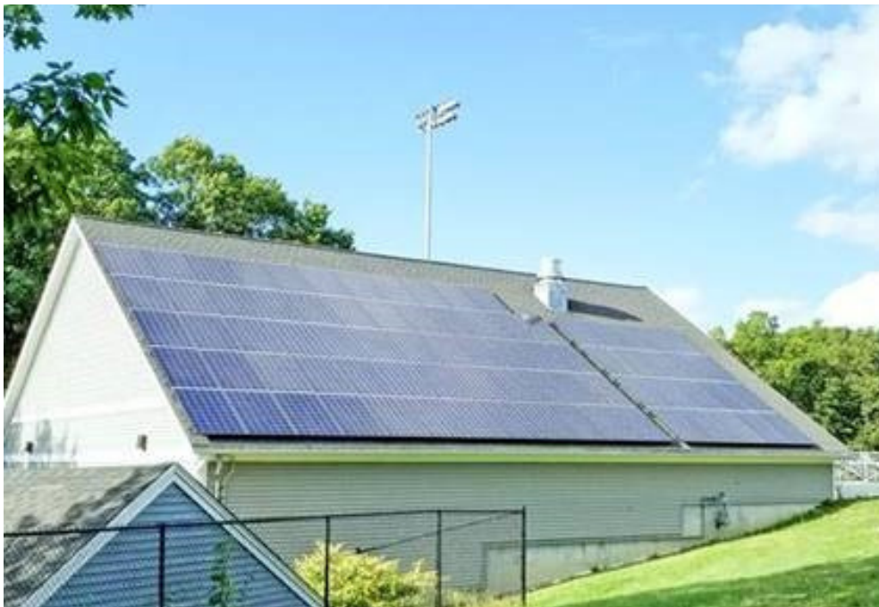
Solar array on service building that was completed in 2017
